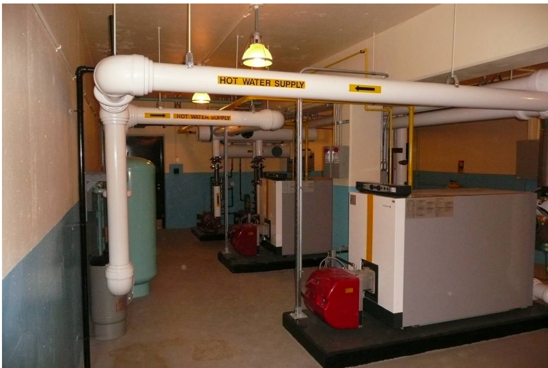
Figure 4: Elgin Water Treatment Plant Boiler Room
