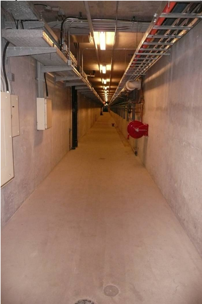
Figure 5: Tunnel at the Elgin Area Water Treatment Plant featuring improved lighting conditions using energy efficient light sources controlled by motion sensors.
